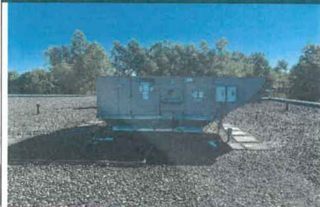
EXAMPLE RTU | PACKAGE UNIT GAS 10 TON
