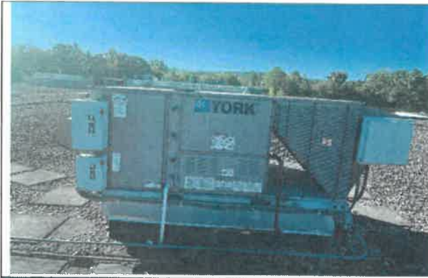
EXAMPLE RTU | PACKAGE UNIT GAS 5 TON
