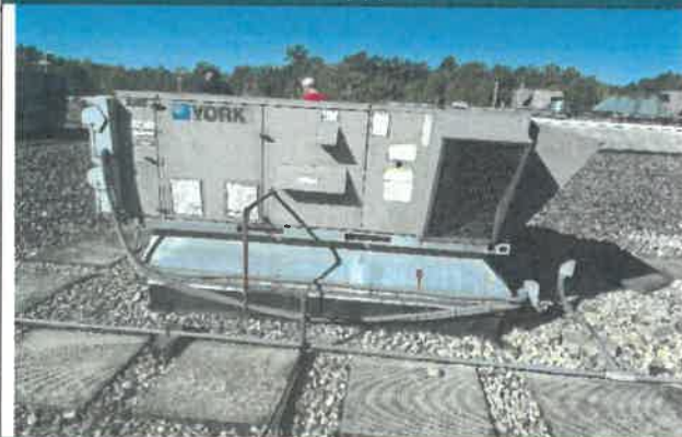
EXAMPLE RTU | PACKAGE UNIT GAS 3 TON
