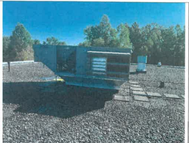
EXAMPLE RTU | PACKAGE UNIT GAS 15 TON
